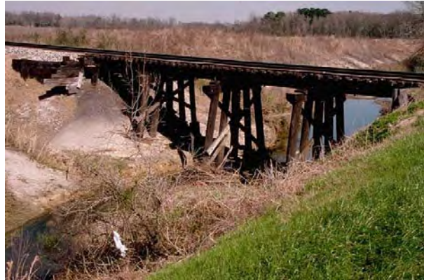
Figure 11. Vegetation around wooden bridges is a serious fire hazard.
