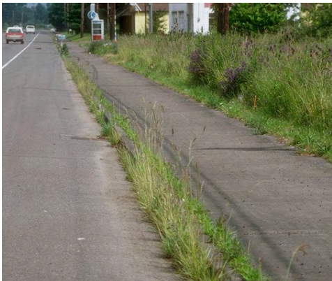
Figure 7. Cracks and crevices support vegetation on roadsides.
