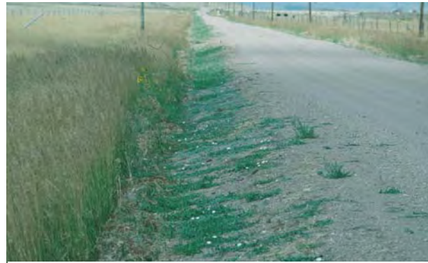
Figure 6. Vegetation on the road shoulder increases maintenance problems.
